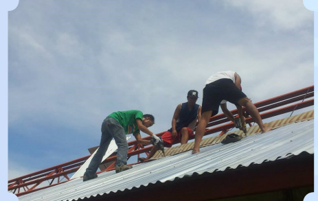
PPMC also contributed in the improvement of SI-BOL/Multipurpose Building in one of the GK sites in La Union as venue for day care session, community gatherings, meetings and trainings.
